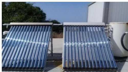
Fig. 2. Evacuated tube solar collectors used in the SWHS.
